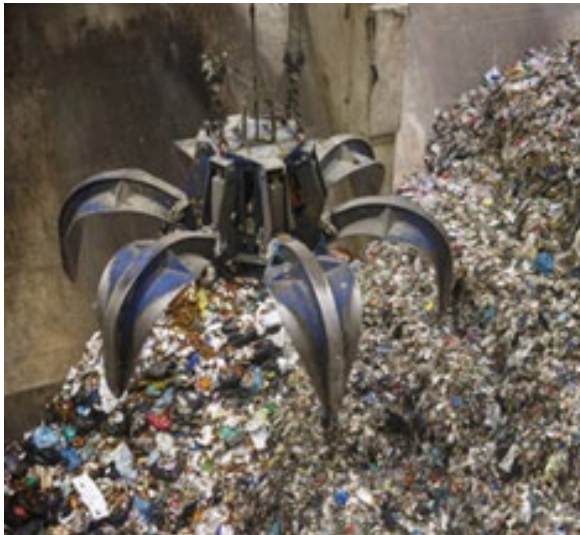
A grab crane operating in a waste storage bunker
