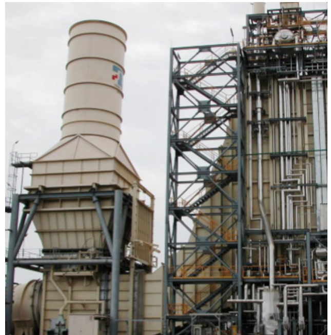
Gas turbine exhaust duct and HRSG at a combined-cycle power station
