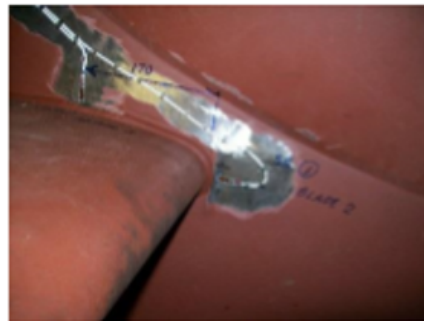
Strain gauging on an ID fan impeller to survey strain during operation
