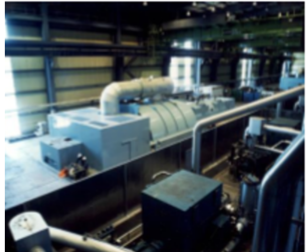
Performance testing of upgraded large steam turbine-generator
